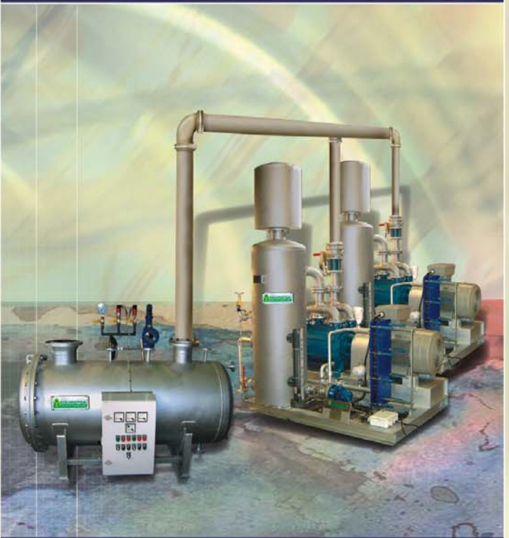
SUCTION PRESSURE: 147 TORR. PRIMING SYSTEM FOR TURBINE CONDENSER IN A COMBINED CYCLE POWER PLANT
